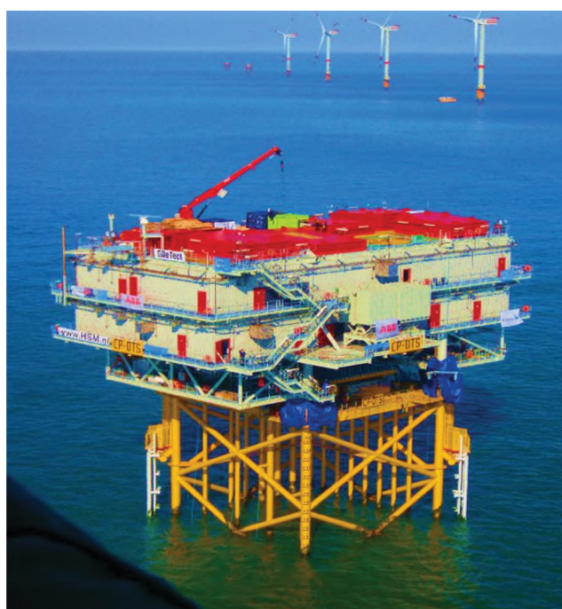
Figure 6. Offshore substation of ABB [8].
